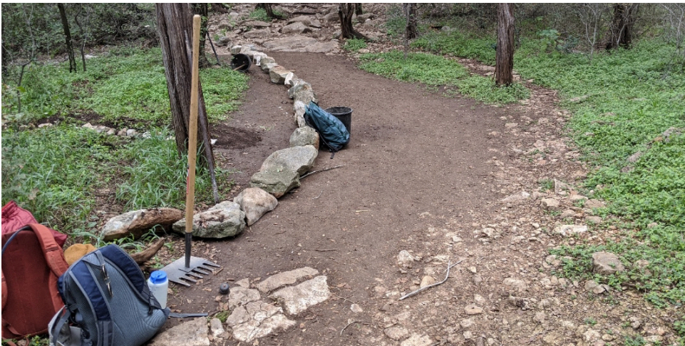
Rocks used to delineate a more narrow path in a wide segment of the trail. ▼
