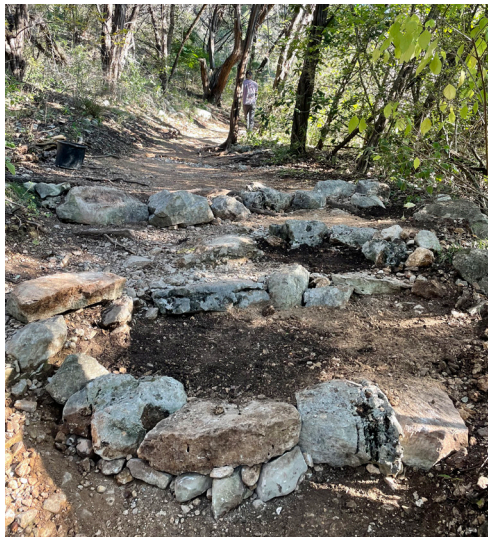
A section of trail that was eroded near the Gaines Creek Trail Head was built back up using local rocks and soil from excavated erosion control trenches. ▶
